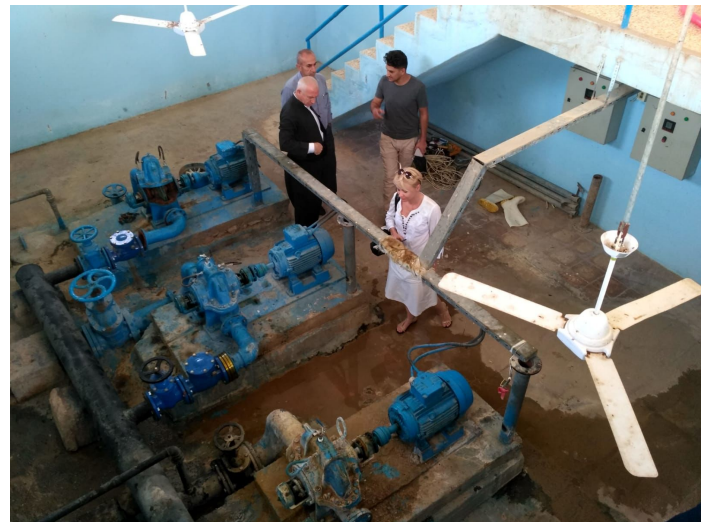
Pumping station in Sheikhan district, Iraq.
